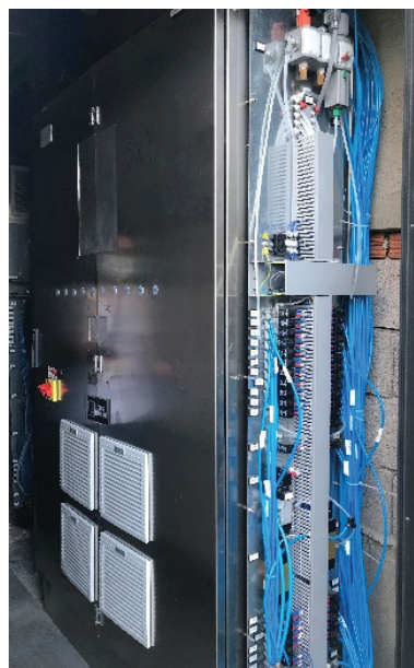
Figure 2. PLC and SCADA system control panel
