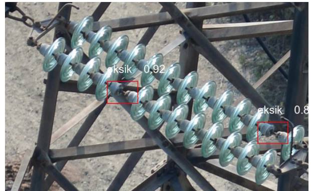
Figure 6: Detection of bird nest fault
