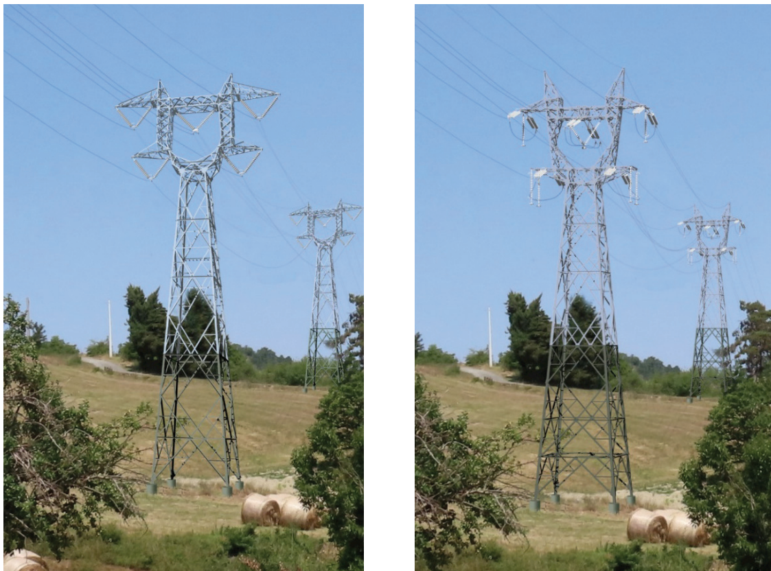
Figure 1. Suspension (left) and anchor (right) towers for “5-phases”
