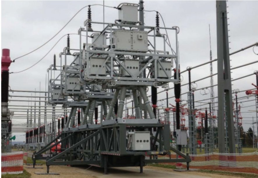
Figure 6: Mobile SSSC device installed in substation
