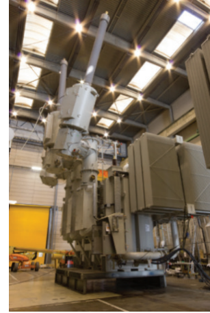
Assembled in Transformer
