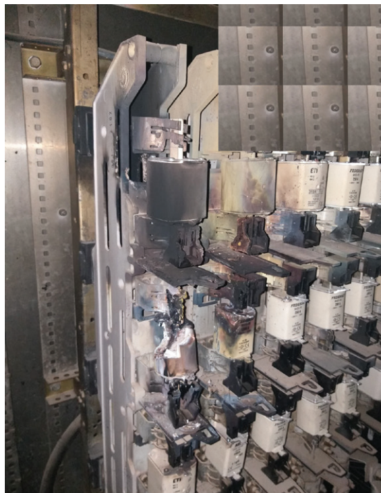
Figure 8. LV fuses blown as a result of overload
