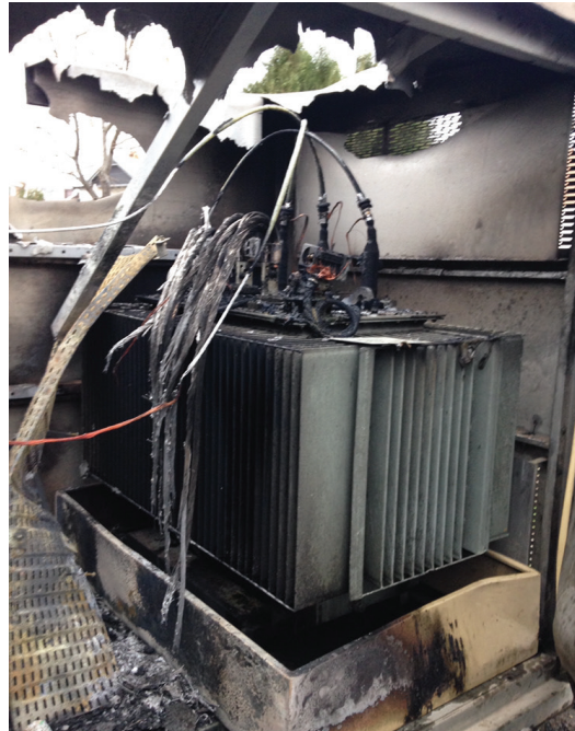
Figure 7. 10/0.4 kV transformer burnt due to overload
